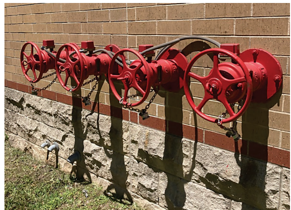
Top: Vulnerability research is a requirement for proper flood protection. Above: Above-grade building penetrations must be identified and protected.
