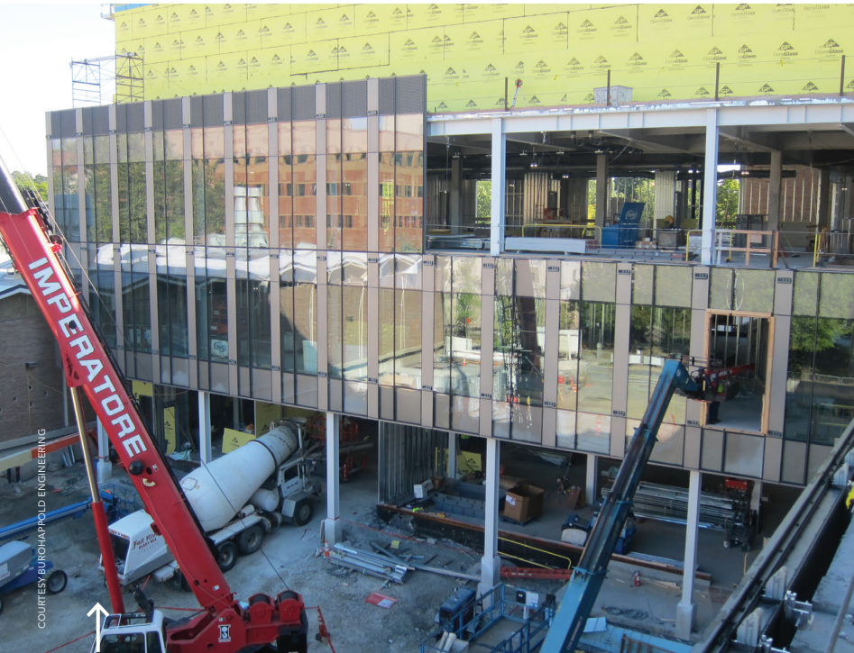
The engineering labs employ a metal decking with hangers and acoustic roof decks to provide versatile setups as well as sound isolation, vertical and horizontal load resistance, and a means of affixing piping, ducts, and other utilities.
