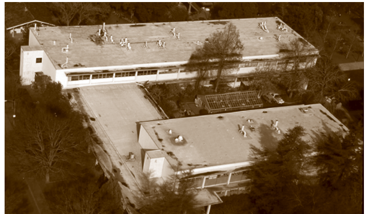
The Sarnafil roofing system that UC Davis chose in 1981 has been protecting critical learning spaces at Robbins Hall for more than three decades.
