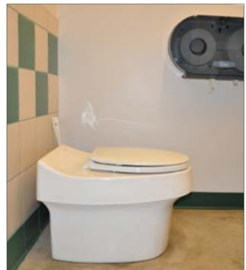
Composting toilet at University of British Columbia's C.K. Choi building.
