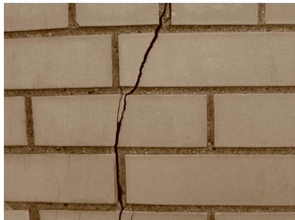
Vertical crack in a glazed brick façade. A major characteristic of Modern buildings was the shift from façades with thick, massive walls and proportionally few windows to slimmer wall construction and more widespread use of glass.
