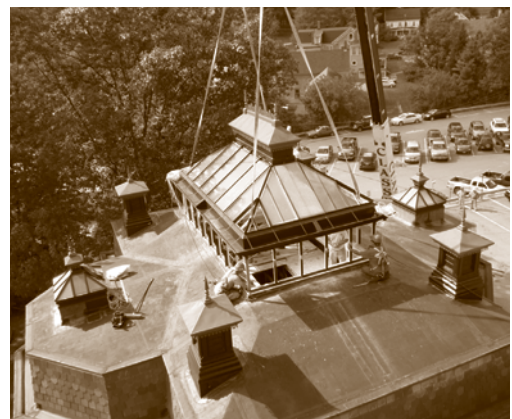
Installation of the skylight at the Athenaeum in St. Johnsbury, Vt. The electronically controlled dynamic glass controls the amount of daylight entering the interior of the art gallery.
