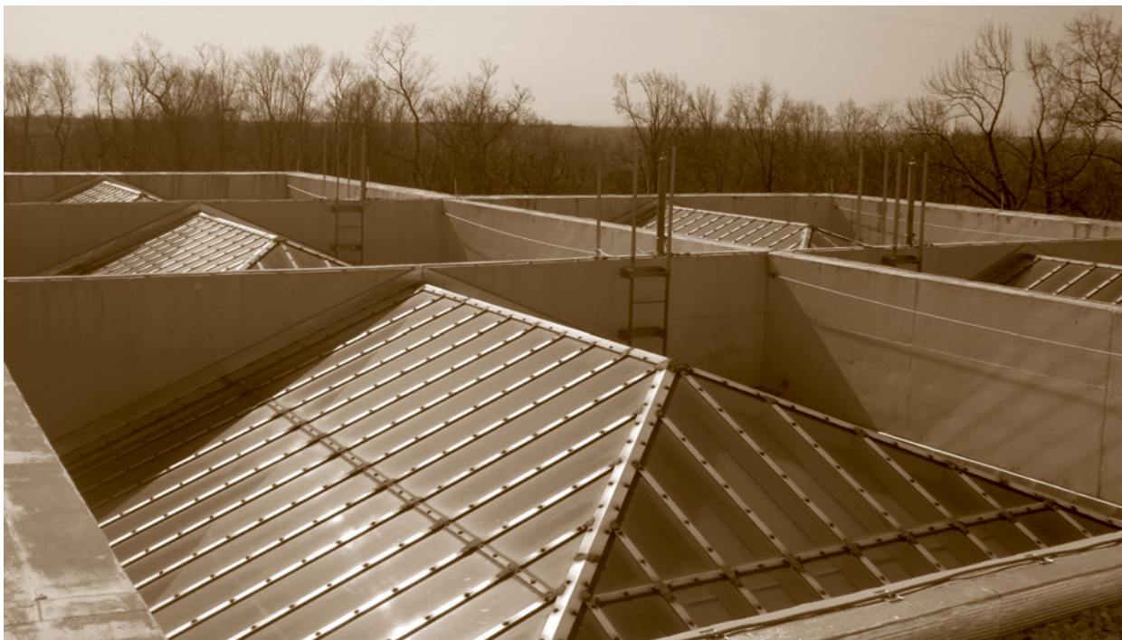
An integral part of the balance of light and mass in many Modernist buildings, skylights are also notorious for leaks, condensation, and poor energy performance. Modernist buildings face a unique threat in that Modernism's break with the artistic styles that preceded it have called into question current perceptions of the historical value of these structures. "The perceptions of one time period with respect to the previous one are often reactionary and, to some extent, negative," according to Bradley T. Carmichael, PE.
