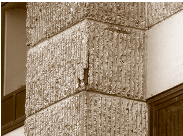
Reinforcement corrosion and spalls in béton brut (“raw” concrete), an aesthetic feature commonly used by architects of the Brutalist tradition, among them Paul Rudolph. His Art + Architecture Building at Yale University recently underwent a major renovation.
