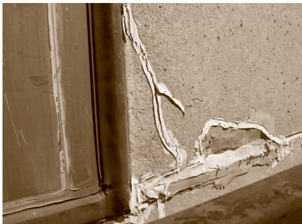
An inappropriate crack repair using surface-applied sealant. Many Modernist buildings used materials and construction techniques that are susceptible to long-term degradation due to corrosion, rot, mold, and ultraviolet radiation.
