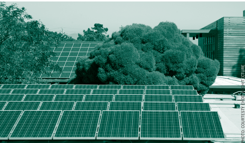
Marin Country Day School, Corte Madera, Calif., a 23,094-sf NZEB powered by a 95.5 kW PV array. Natural ventilation, cold water storage, solar shading, daylighting, and occupancy sensors were used to keep energy consumption to a minimum.
